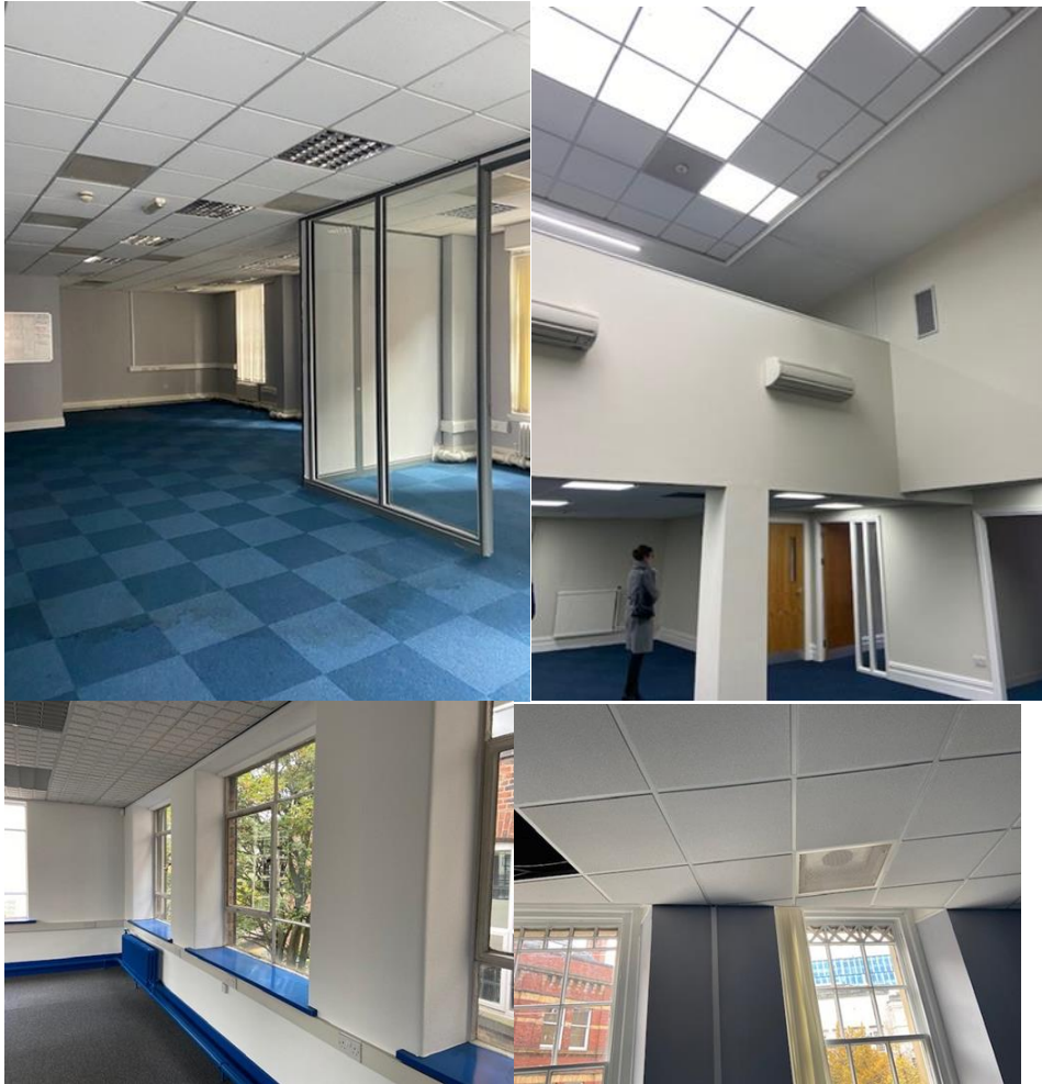
Photos c) d) e) f) and g) The existing interior of Reedham House
